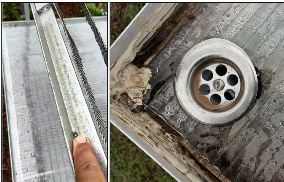
Fig. 54. Water leaking and tray breakage issues observed in the field deployed i-FWC 2.0.
